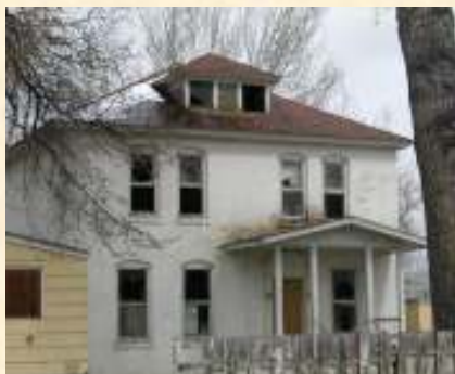
A Piece of History —The restoration of this historical building on the Crow reservation is slated as a future Operation Walking Shield project.
